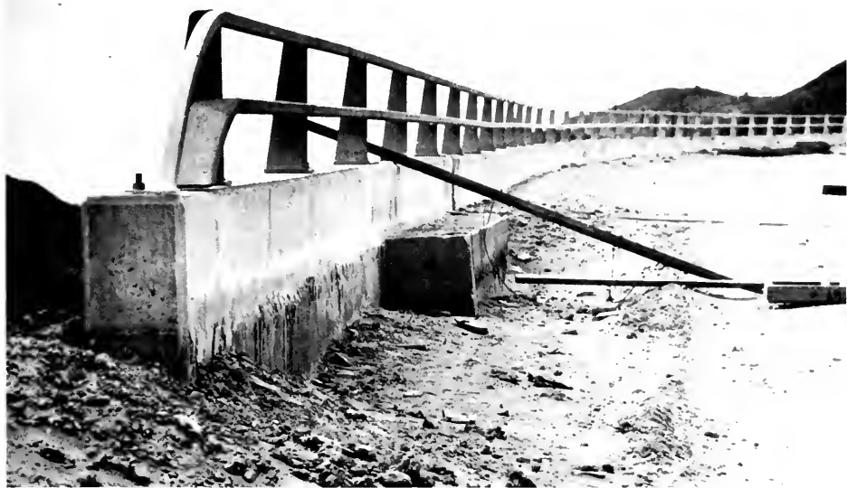
Photo 20. Settlement of backfill at abutment of overcrossing at the Golden State Freeway and State Highway 14 interchange [7].
